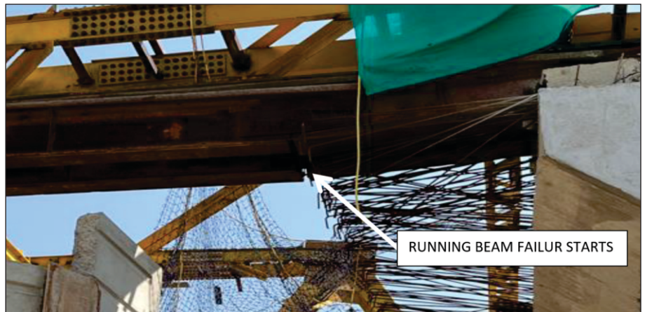
Fig. 5 : Photograph of Running Beam at Failure Side
