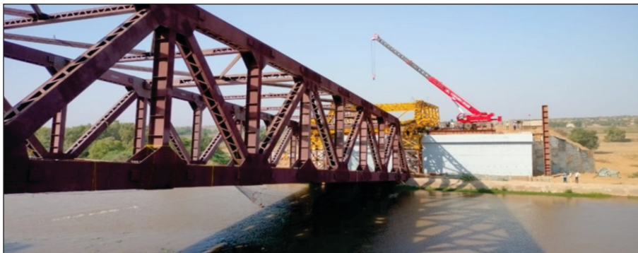
Fig. 4 : Photograph Showing Collapse of Main Truss Launching End
