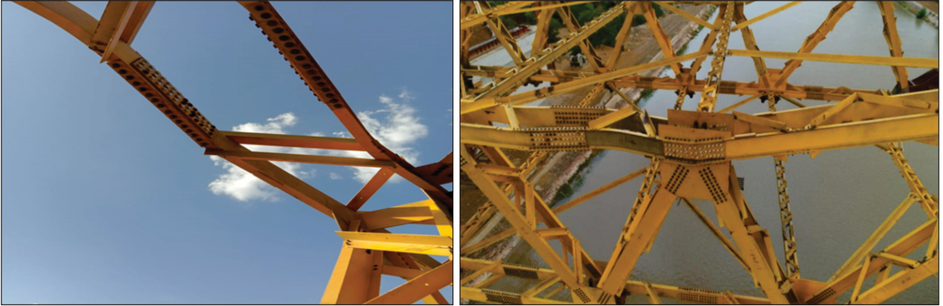
Fig. 3 : Photograph Showing Buckled Top Chord of Nose
