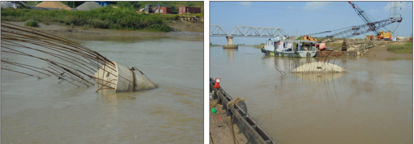
Fig. 3 : Excessive Well Tilting
