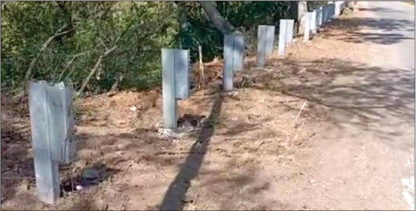
Fig. 2 : Missing metallic crash barriers along a state highway
