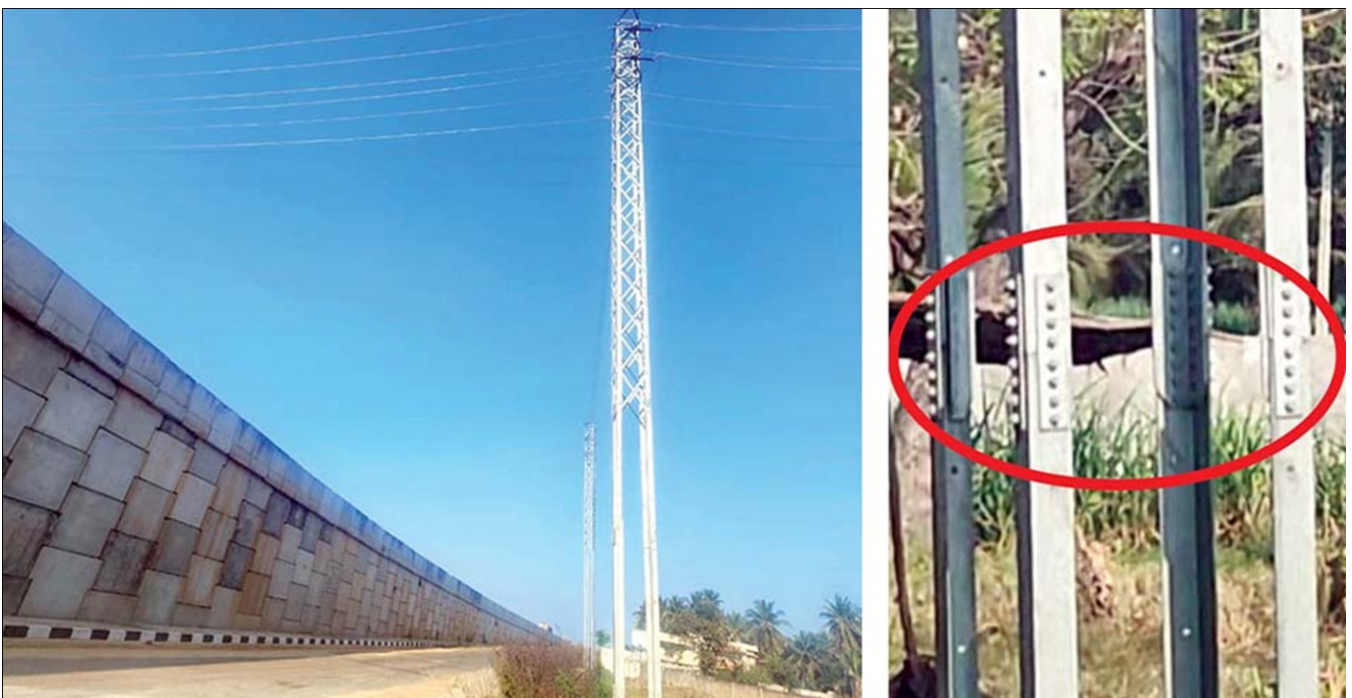
Fig. 3 : Missing lacings and battens in electric poles along the Expressway
