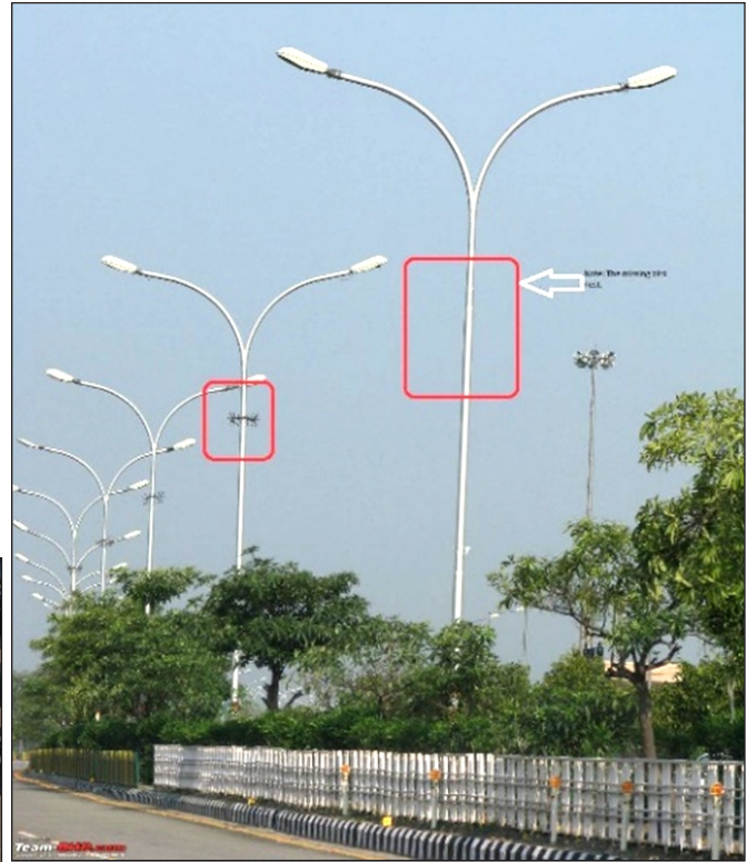
Fig. 4 : Missing Bird's nest in electric pole
