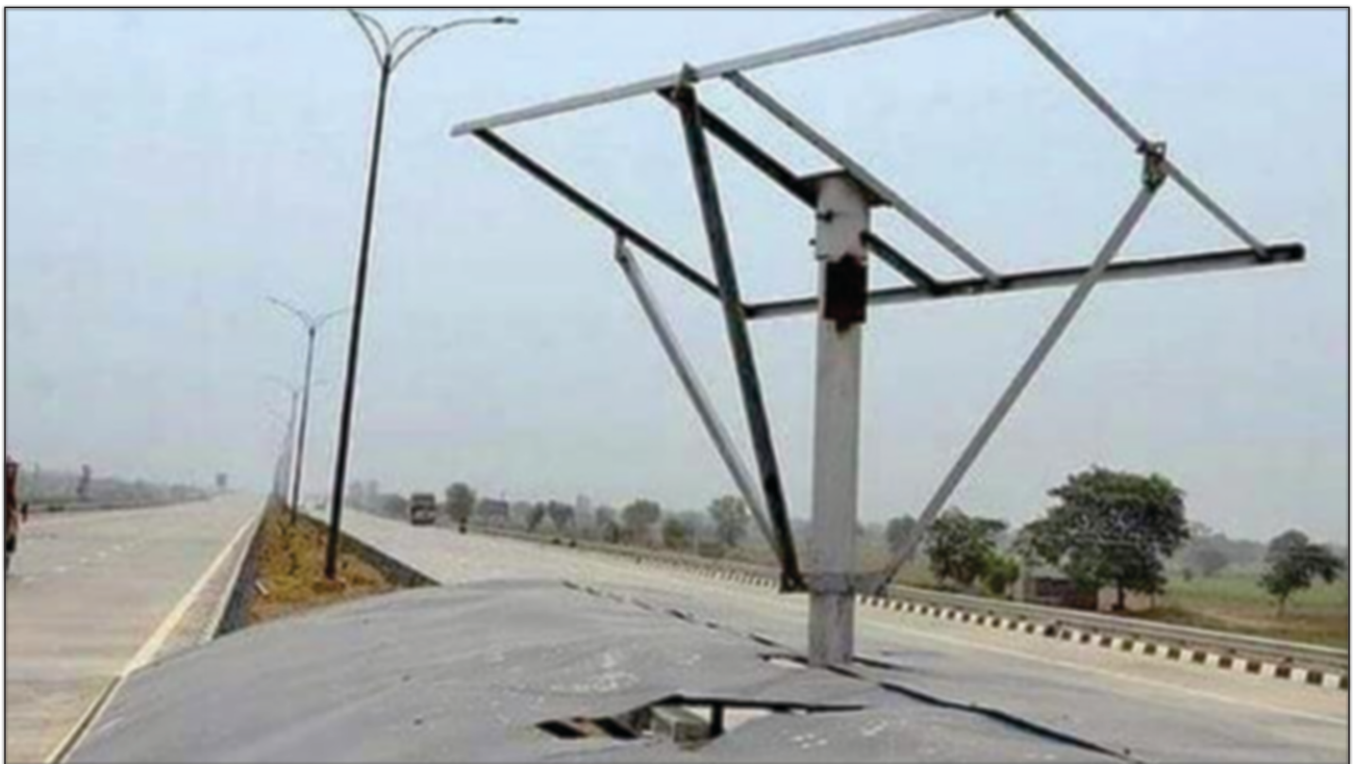
Fig. 1 : Missing solar panels along the Expressway (pic via Twitter)
