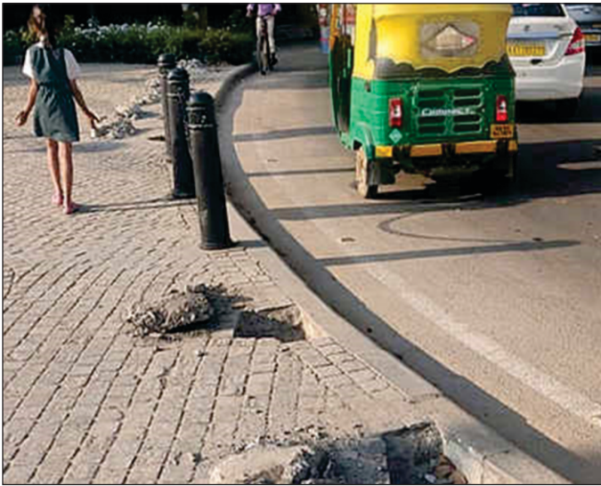
Fig. 5 : Bollards stolen despite CCTVs near the traffic island
